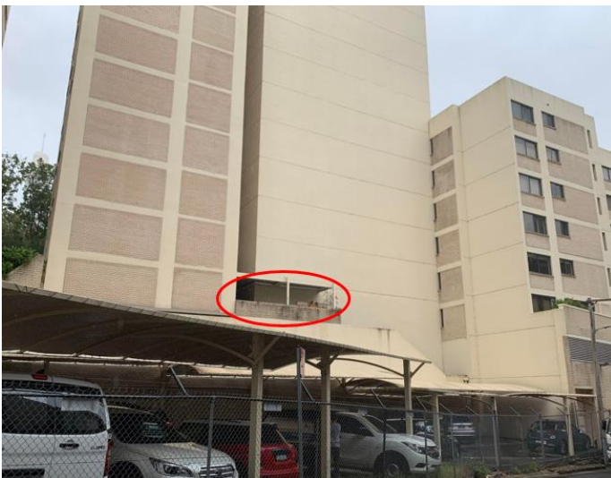
Figure 29: Existing eastern facing balcony of an apartment within 1 Boomerang
